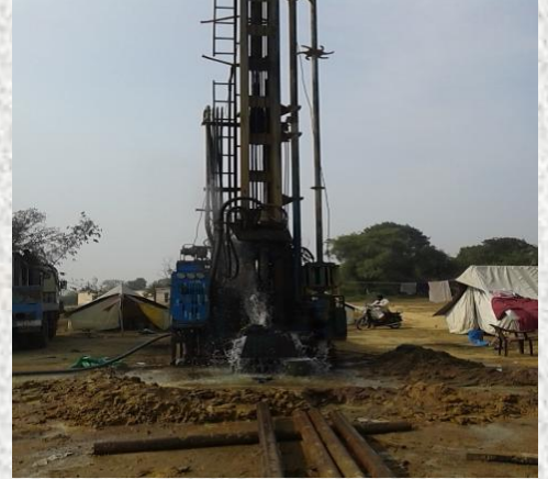
DTH drilling of EW at village Bedia of Jama block, Dumka district
